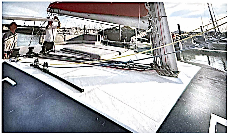
Custom solar panels installed on the coachroof.
