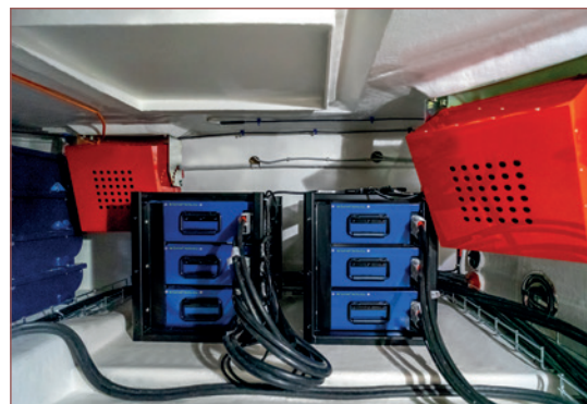
The Sunreef monitoring system allows you to check all the data on board, such as the readings from the thermal cameras.
